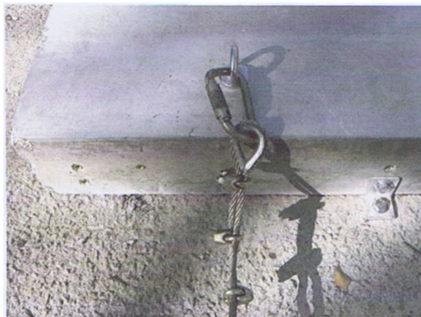
Figure 1 – Anchor device described as “Concrete anchor”
