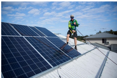
Figure 4 Incorrect use of rope systems can lead to massively increased risks
