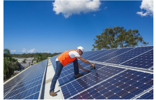
Figure 1 Incorrect safety provision for maintenance workers is wide spread
