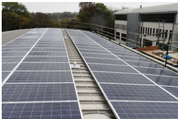
Figure 6 Panels and Lifelines positioned for ease of access
