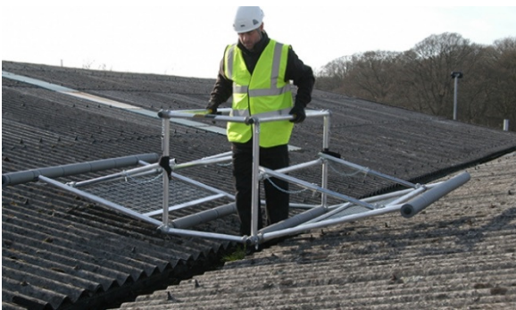
Figure 6 Mobile Barrier systems employed to allow gutter access for maintenance
