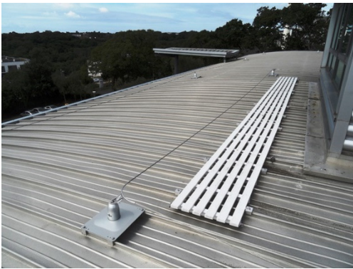
Figure 1 Walkway and Lifeline for window and gutter access
